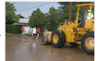
Heavy equipment and volunteers help clear the road in Nogales after Friday's storm. Photo by Manuel C. Coppola/Nogales International
